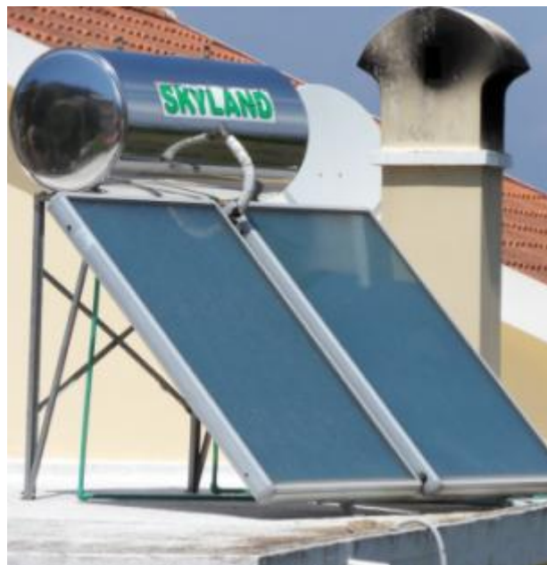
Figure 2.3: Pressurized System with Horizontal Storage Tank in Greece
