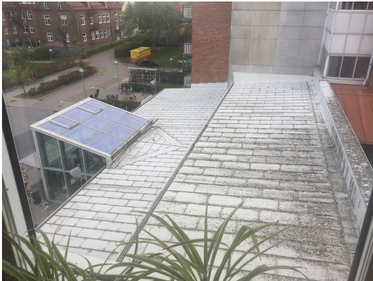
Image 5. View to the roof over the main entrance from the elevator hall at the fourth floor (left).
