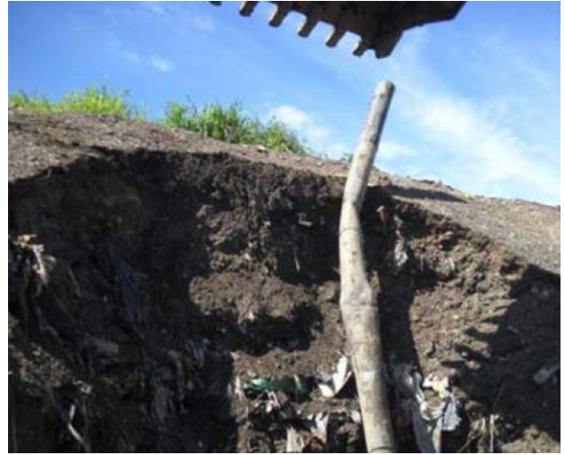
Fig. 4. Temporary covering of non hazardous waste dump with engineered material arising from mixed soils, glass, debris from clean water sedimentation (credits Oggeri 2014).
