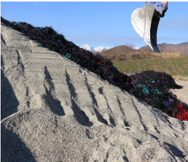
Fig. 2. Two types of non-conventional materials: the slope in the foreground is made of different fragmented and sieved glass; the bench in the background is made of polymeric cuttings from gasket production (credits Oggeri 2019).
