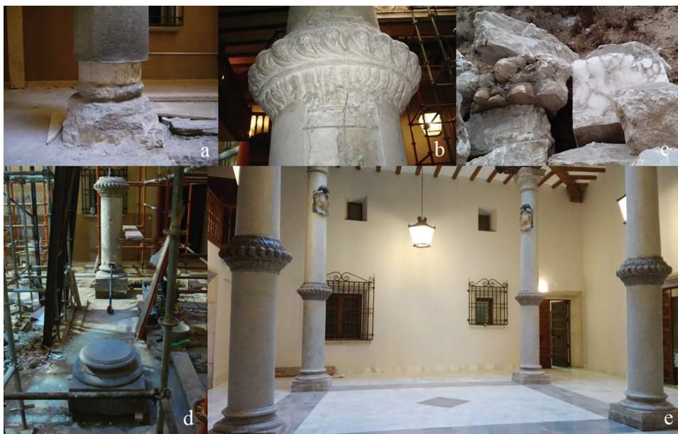
FIGURE 1. a. Removal of mortar on base. b. Removal of reinforcement mortar that covered lower part of carved ring and shaft. c. Alabaster quarry. d. New bases. e. Restored alabastrine gypsum columns.
