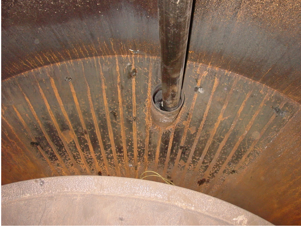
Figure 1-1. Accelerated corrosion in the breaking strips where strain is concentrated.
