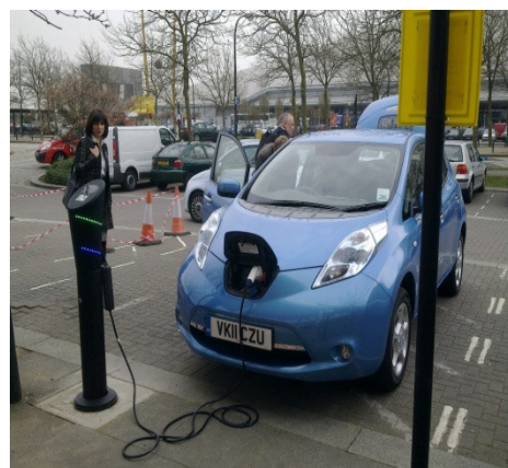
Figure 6.4: The first EV charging point in Milton Keynes. The point was installed for the Nissan leaf launch in Central Milton Keynes in March 2011
