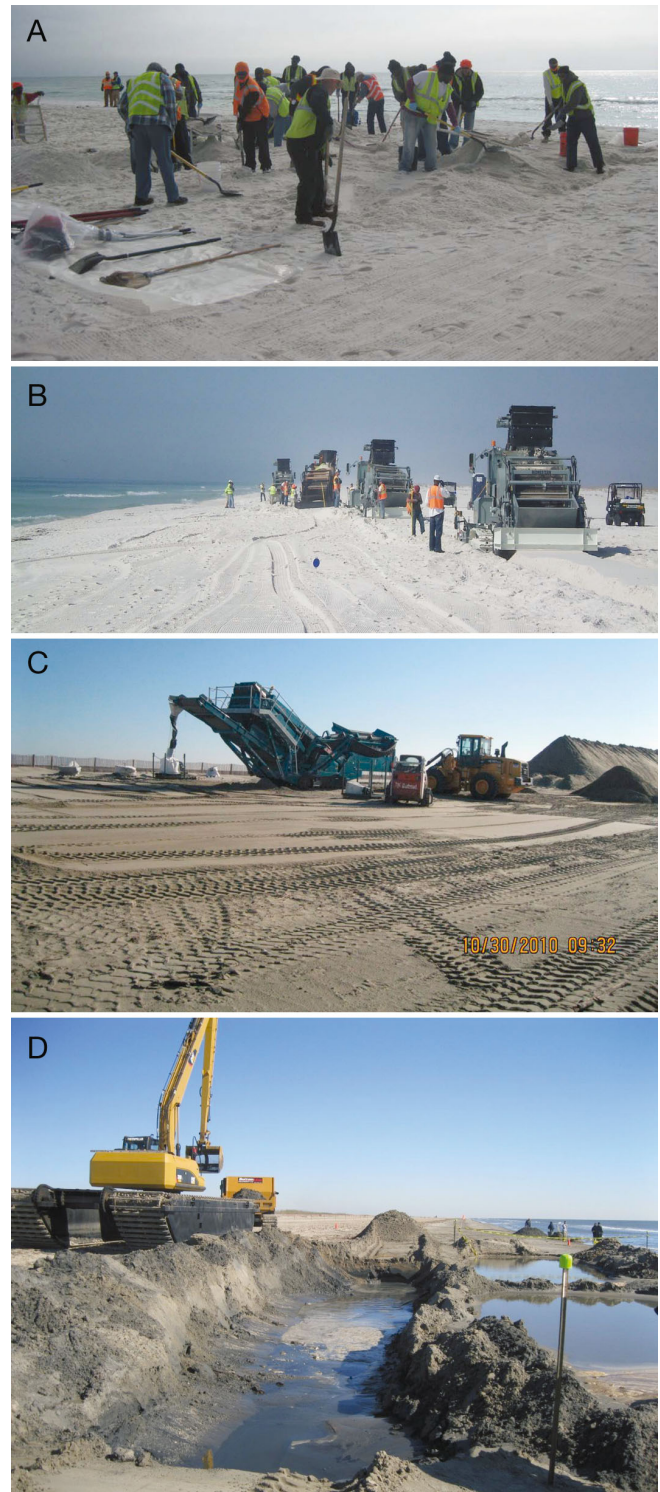
Fig. 4. Sand beach treatment methods. (A) Manual removal/sifting to 15 cm at Ft. Pickens, Florida, January 2011. (B) Four 'Sand Sharks' at Ft. Pickens State Park, running in tandem and sifting to 45 cm, February 2011. (C) Sifting of sediment piles created by mechanical removal on Grand Terre II, Louisiana, October 2010. (D) Excavation of oil mats at Elmers Island, Louisiana, December 2010
