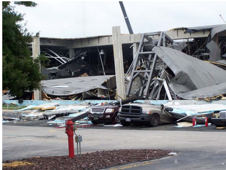
Figure 7: ConAgra Natural Gas Explosion and Ammonia Release 7
