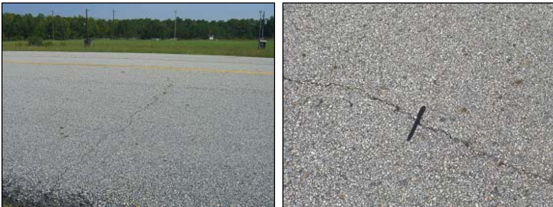
Figure 9 Transverse cracking along Taxiway A at Griffin-Spalding Airport
