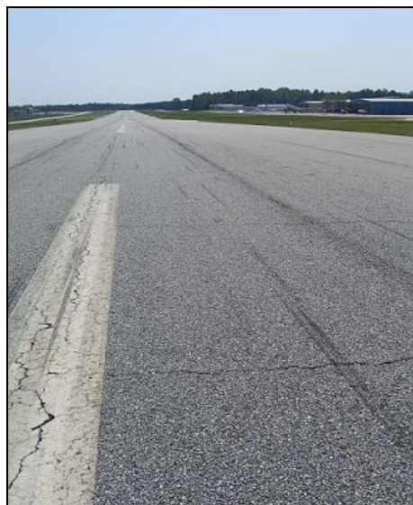
Figure 8 Transverse cracking along Runway 14-32 at Griffin-Spalding Airport
