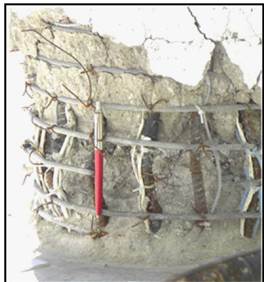
d) Long. Bars and Spiral Rupture
