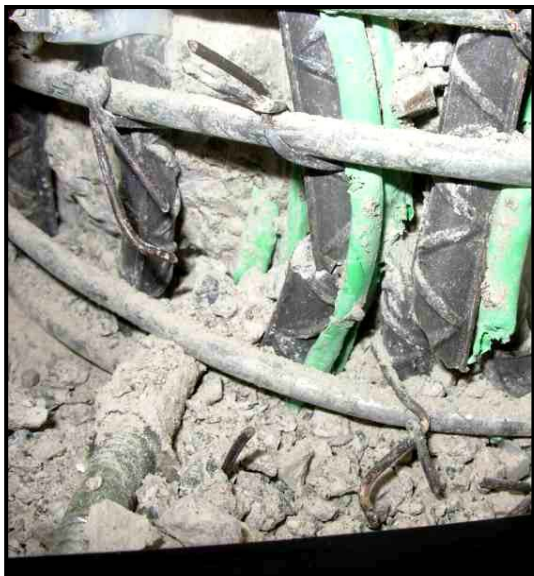
e) Long. Bars Rupture
