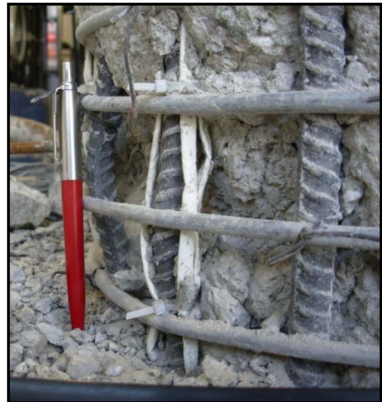
d) Long. Bars Buckling
