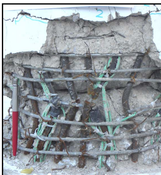
d) Long. Bars and Spiral Rupture
