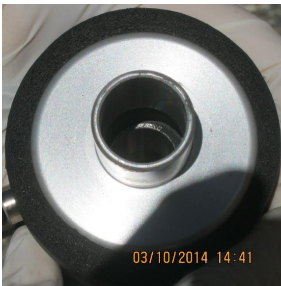
Figure 6: Condensation water trap during a cleaning on October 3, 2014. Black powder was visible in the condensation water trap. The black around the outside of the trap is insulating foam.
