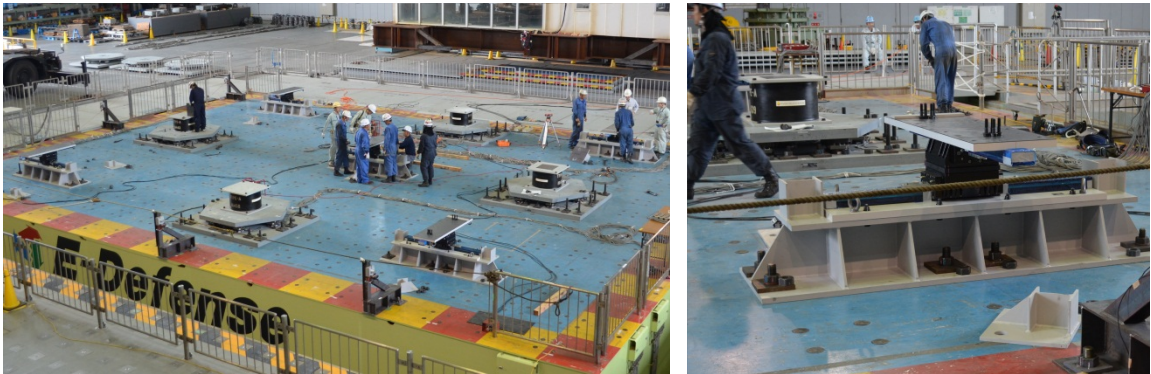
Figure 4-14: Installing the LR bearings to the connecting assemblies and the CL bearings to the simulator platform
