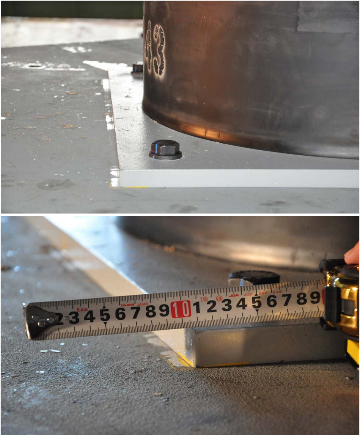
Figure 5-15: Permanent displacement of around 11 mm on the East bearing due to sliding of the bottom steel plate.
