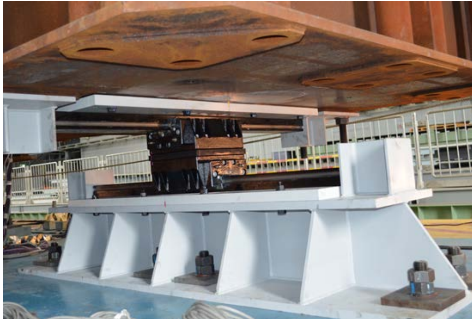
Figure 3-10: Photo of installed CL bearing illustrating orthogonal LM guides assemblies on top and bottom.
