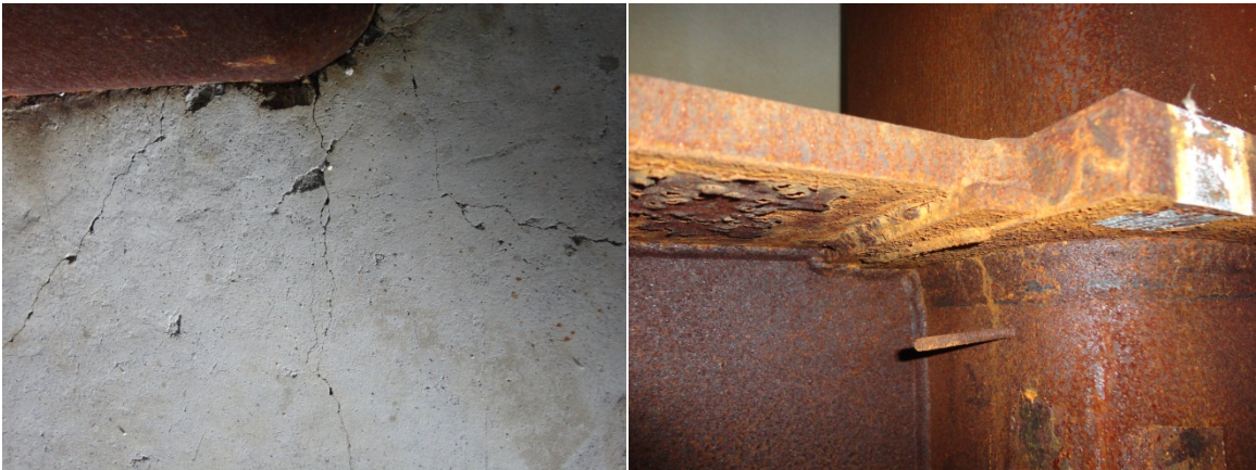
Figure 2-11: Cracks in concrete slab and rust on steel member
