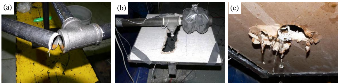
Figure 8: UB Piping Experiment: (a) tee joint rupture, (b) ceiling-piping damage, (c) activated sprinkler head, Source: (Tian et al., 2013)
