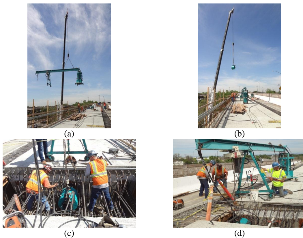
Figure 2-15 Prestressing operational issues: (a) Stressing hoist transfer; (b) Stressing jack transfer; (c) Hinge reinforcement congestion; (d) Hoist stumble
