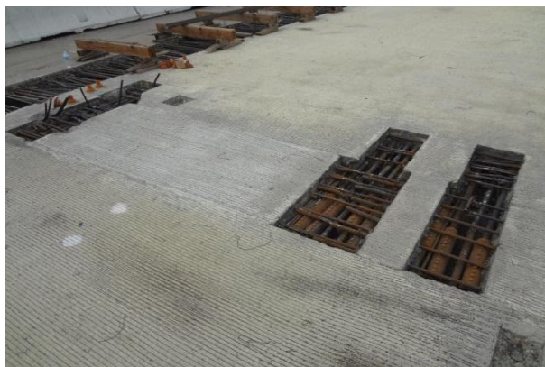
Figure 2-49 Reinforcement steel and couplers connection between Closure 1 and the Segment B of Frame 3, Bridge 5EB
