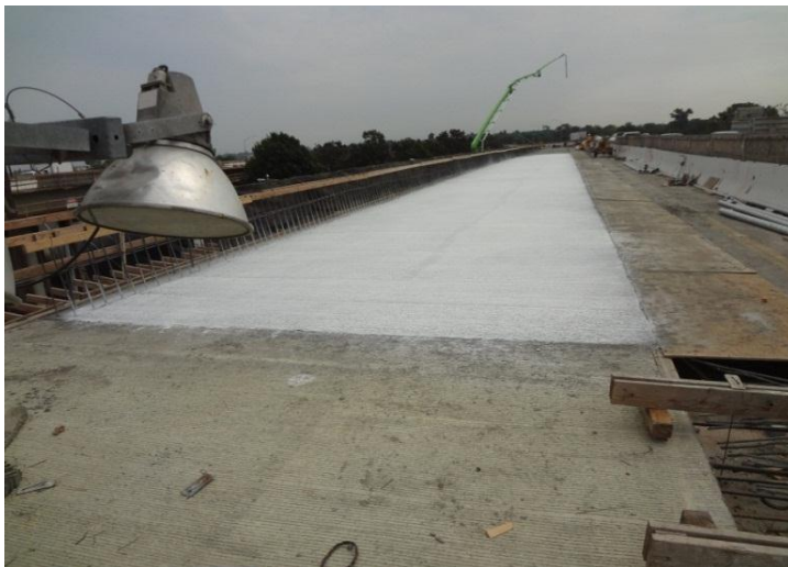
Figure 4-16 Completion of the hinge closure and long cantilever of H1 on Day-68
