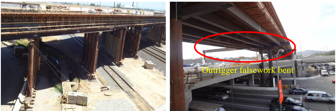
(a) (b) Figure 2-10 (a) Skew falsework bents at Del Paso Park OH; (b) Outrigger falsework bent at Wilshire Blvd
