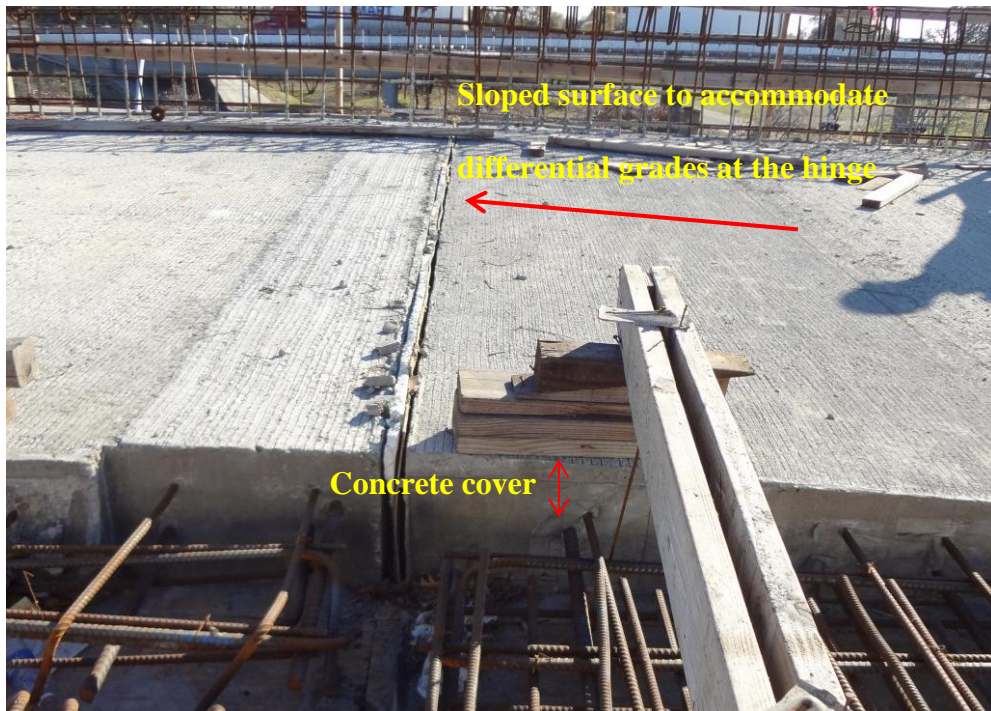
Figure 1-10 Thick concrete cover for top deck reinforcement, Del Paso Park Overhead, Sacramento
