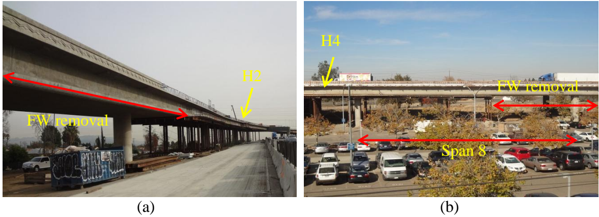
Figure 2-11 Partial falsework removal at: (a) N170-N5 Connector; and (b) Del Paso Park OH
