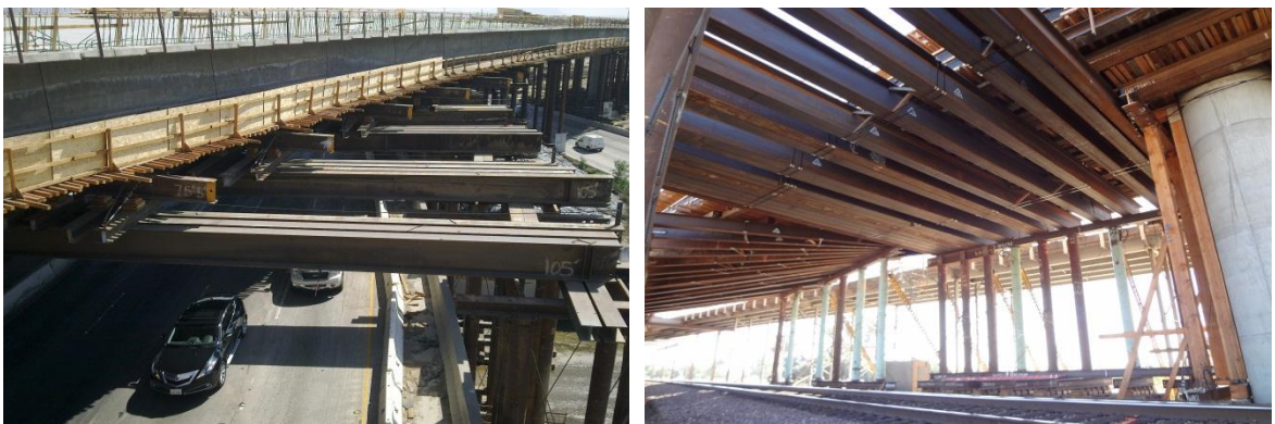
(a) (b) Figure 2-9 Falsework spanning over: (a) roadway at N170-N5 Connector; and (b) railway at Bradley Overhead
