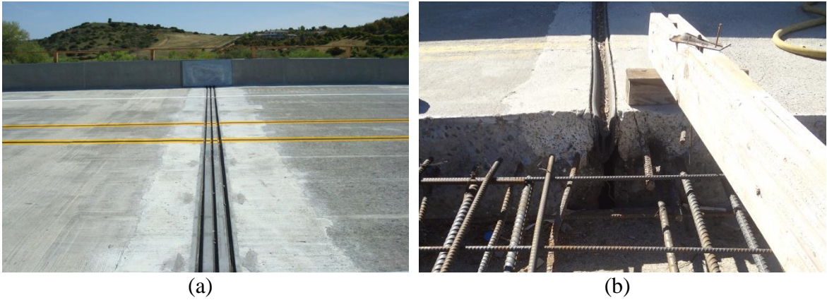
Figure 2-6 Deck joint seals after installation: (a) Joint seal assembly; and (b) Bonded joint seal
