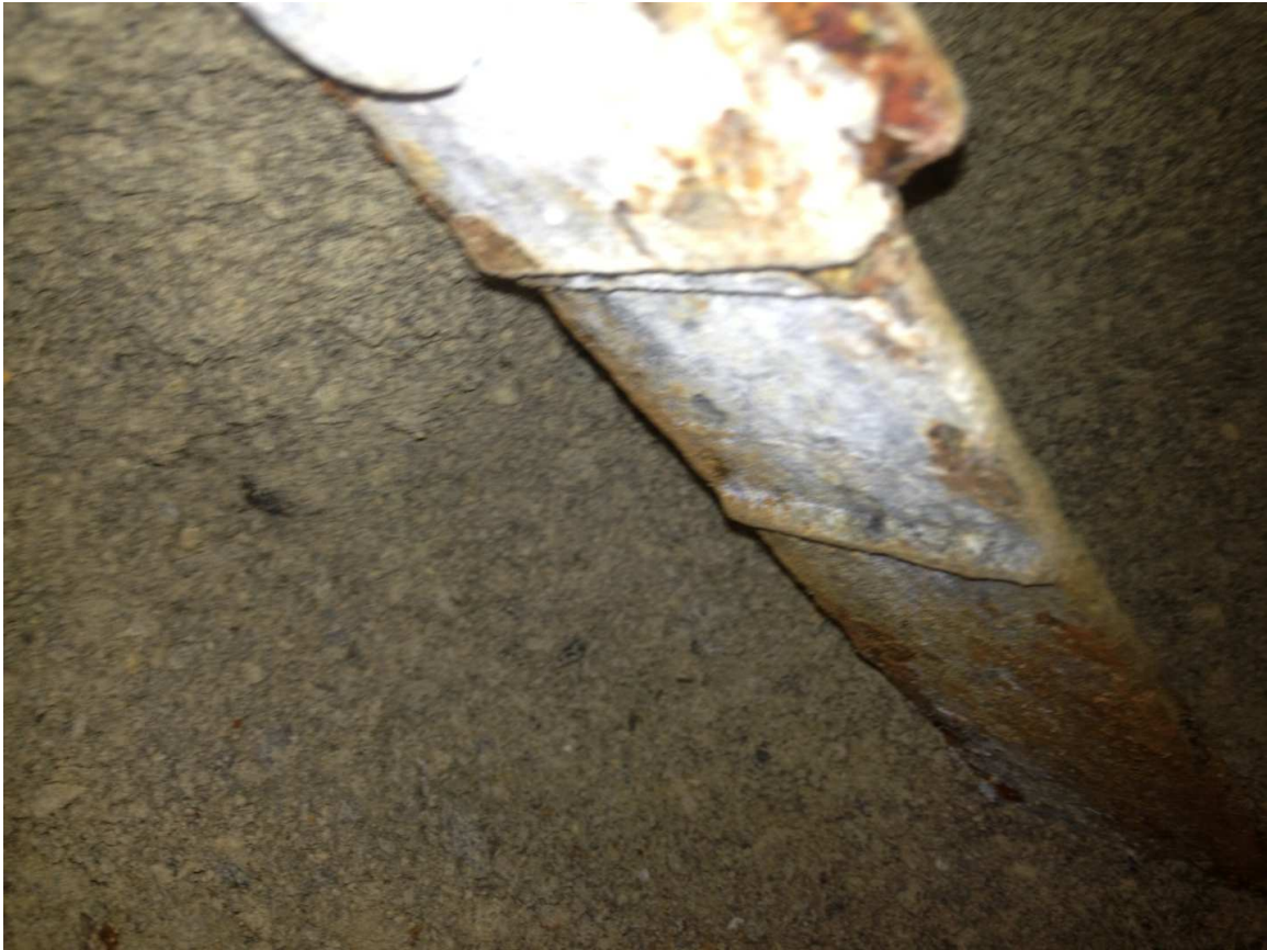
Figure 3-12: In-service galvanized soil reinforcement for I-15/ Cheyenne Blvd. Wall 1, 15 years old.
