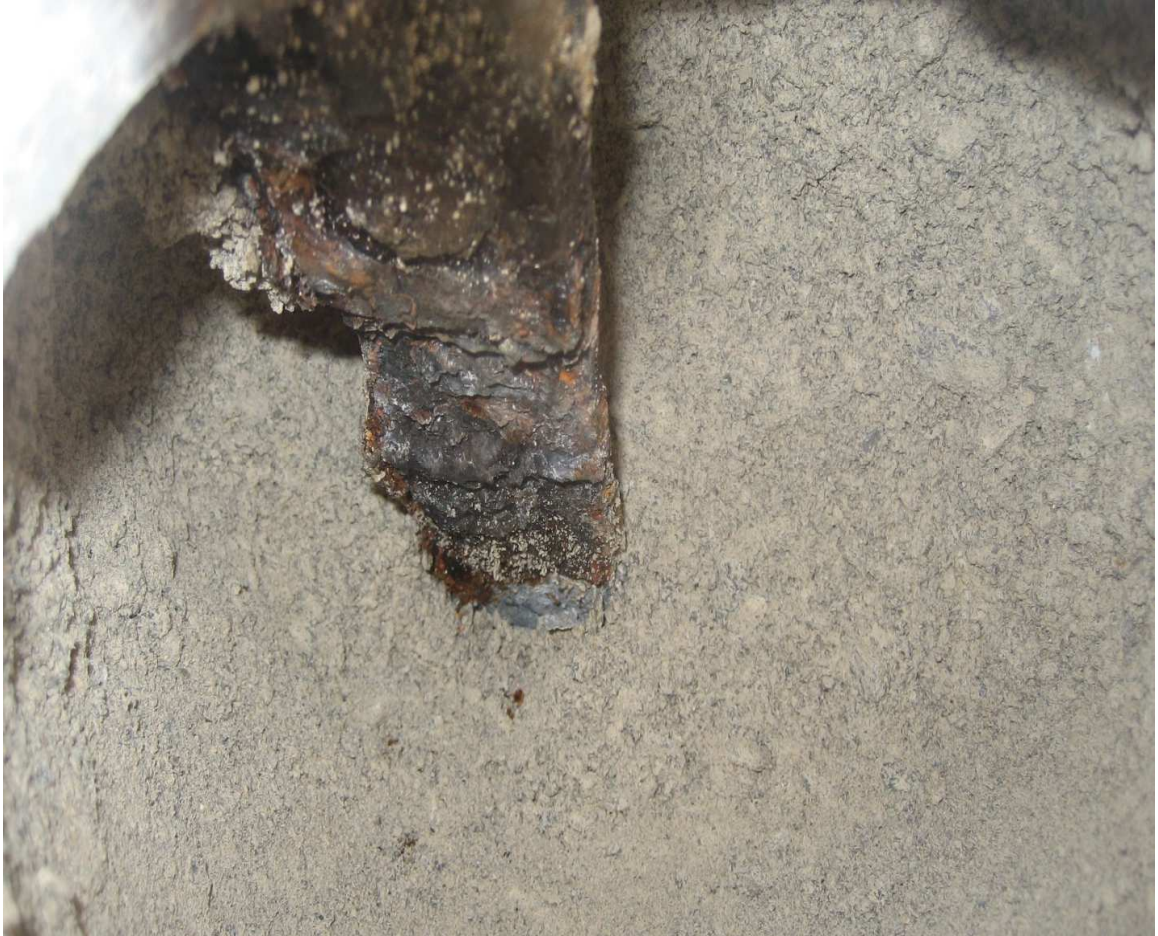
Figure 3-14: In-service galvanized soil reinforcement for I-15/ Cheyenne Blvd. Wall 1, 15 years old. (E1)
