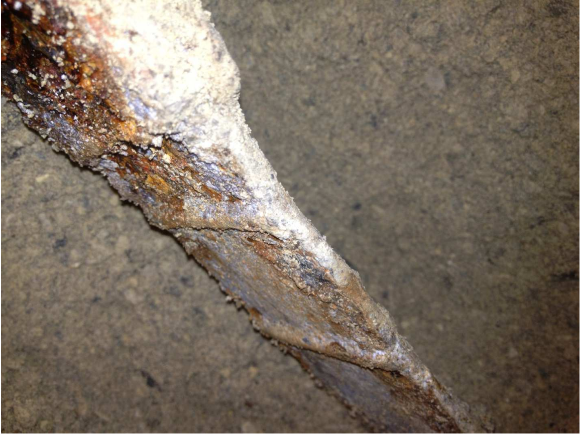
Figure 3-16: In-service galvanized soil reinforcement for I-15/ Cheyenne Blvd. Wall 1, 15 years old.
