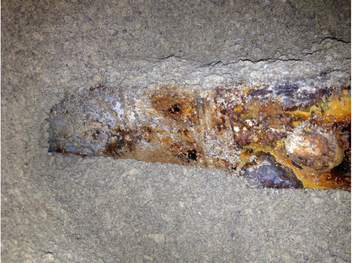
Figure 3-13: In-service galvanized soil reinforcement for I-15/ Cheyenne Blvd. Wall 1, 15 years old.
