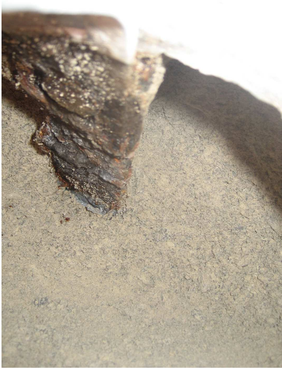
Figure 3-15: In-service galvanized soil reinforcement for I-15/ Cheyenne Blvd. Wall 1, 15 years old. E2)
