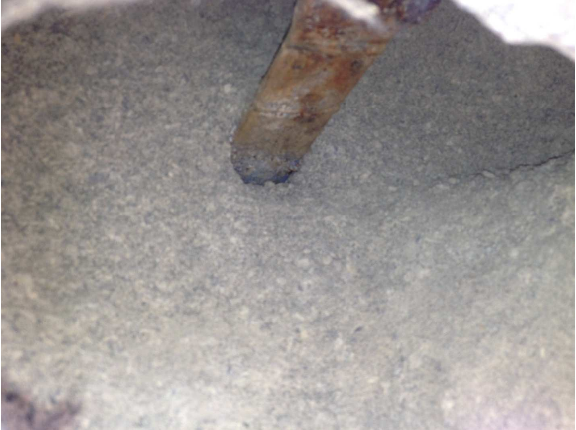
Figure 3-17: In-service galvanized soil reinforcement for I-15/ Cheyenne Blvd. Wall 2, 15 years old.
