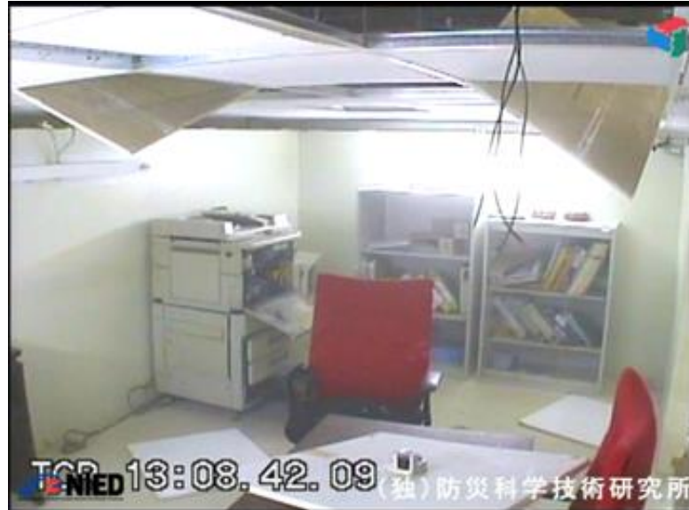
Figure 1.5. Fallen ceiling panels and content disruption in a base isolated building subjected to 80% Tabas (PGA=0.87g horizontal, 0.59 g vertical).
