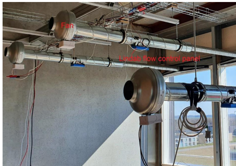
Fig. 6. The exhaust fans for the ventilation system.
