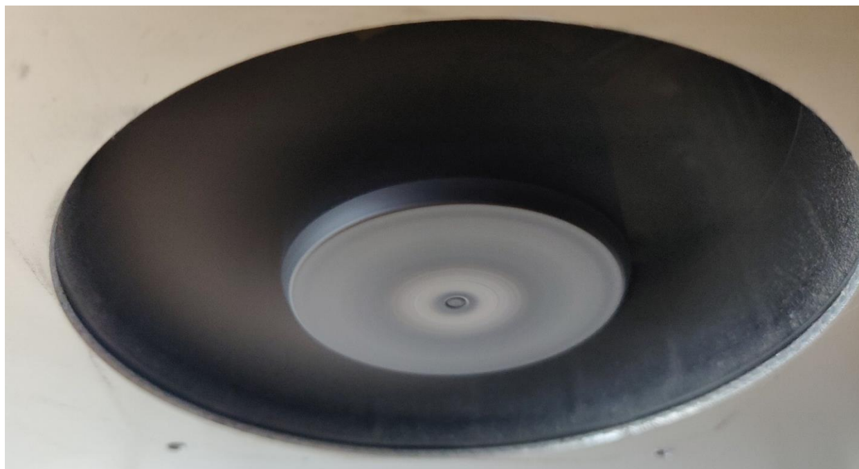
Figure 13: Ventilation fan spinning correctly.
