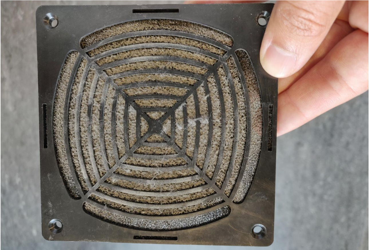
Figure 14: Dirty bottom ventilation filter.
