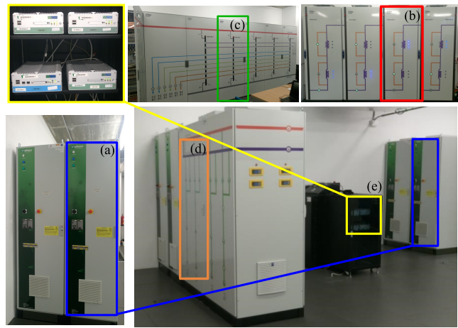
Fig. 9. Photograph of the laboratory facilities. (a) VSC, (b) configurable impedances, (c) AC bus-bars, (d) DC bus-bars, and (e) embedded computers.
