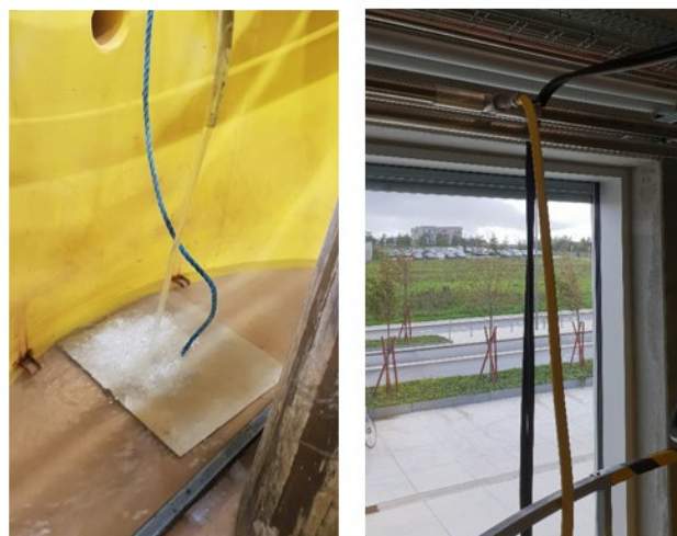
Fig. 4.7. A plate on soil surface for filling the water and water connection from the working platform
