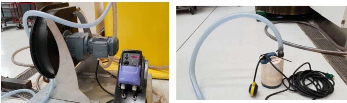
Fig. 3.7. The suction pump and the setting switchboard for the pump (left picture) and the small pump (right picture)
