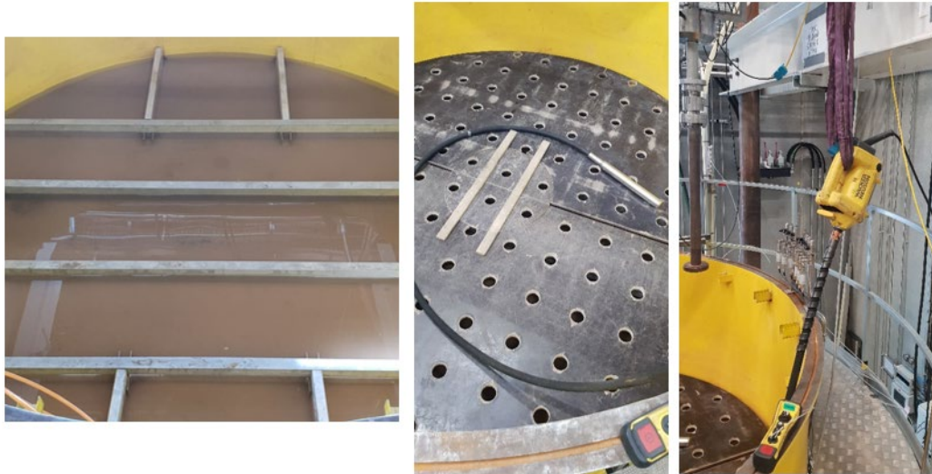
Fig. 4.1. The vibration procedure: the beams below the platform, the vibration platform and the vibrator hanging on the crane
