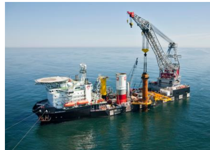
A vessel used for installation of piles for offshore wind turbines ( www.cape-holland.com ).
