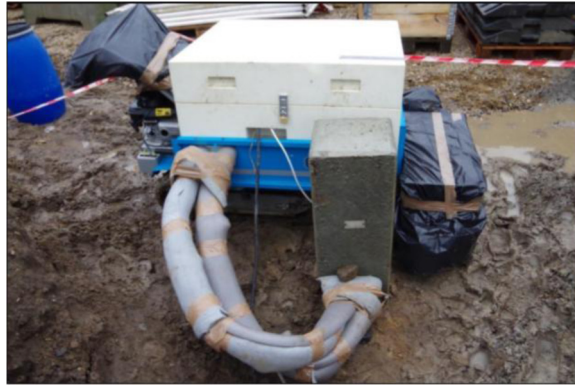
Fig. 1. Ongoing TRT at Langmarksvej. Inlet- and outlet pipes are insulated to prevent disturbances from ambient temperature conditions [2].
