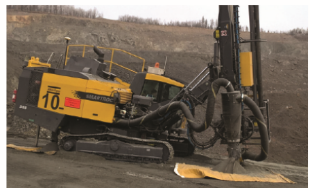
FIG 5 – Experimental drilling with canvas placed under the back discharge and canvas plus sectorial cutter placed under front discharge of the Atlas Copco D65 drill rig.
