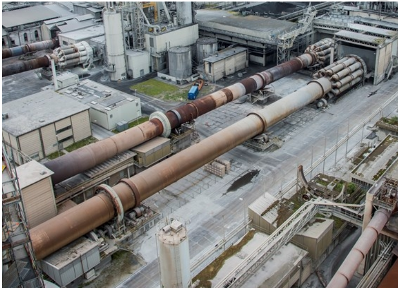
Fig. 1: A view of cement rotary kiln in Aalborg Portland cement factory, Aalborg, Denmark
