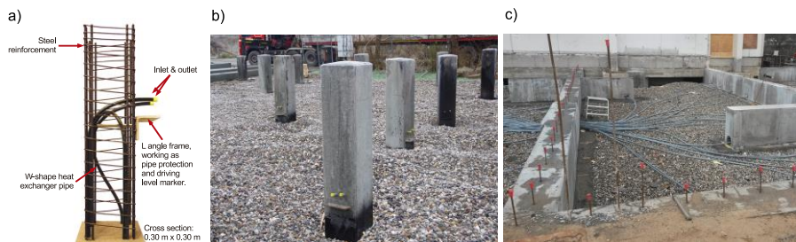
Figure 1: a) Demonstration model of the precast pile heat exchanger with built in geothermal pipes. b) Pile heat exchanger field after driving. c) Pipe work.
