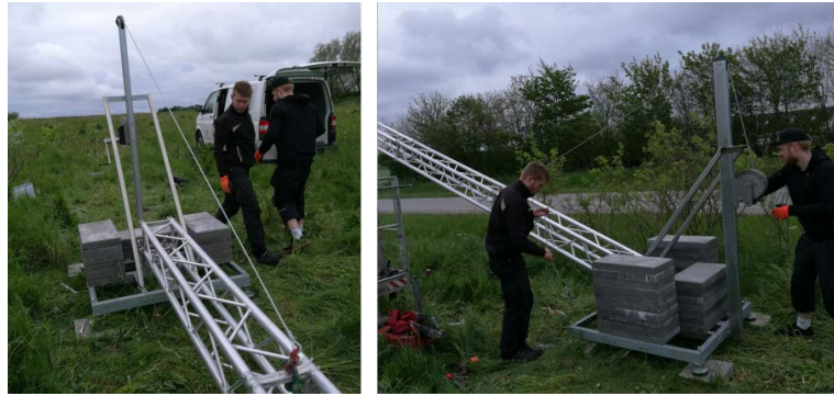
Figure 13. The portable pole can be raised using a swivel bracket installed in the middle of the base platform. The pole is raised using a steel wire connected to a manual winch system.
