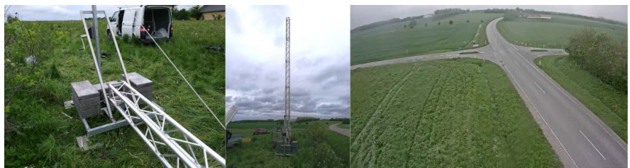
Figure 16. The TRG-pole is deployed at a traffic intersection with limited existing infrastructure.
