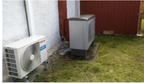
Fig 4: An air to water heat pump at one of the participating households.
