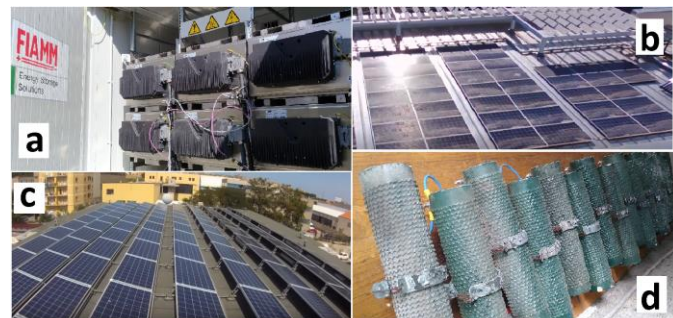
Fig. 4. a) FIAMM storage; b) PV1 generating unit; c) PV2 generating unit; d) adjustable load
