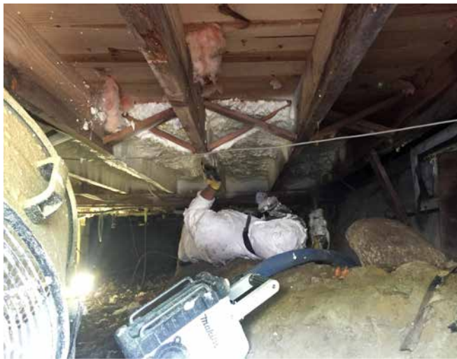
Figure 3.1 Spray foam insulation of (A) a new building (open-cell type) and B) the basement of an old house (also open-cell). The second worker in (A) is trimming the foam with a blade saw.
