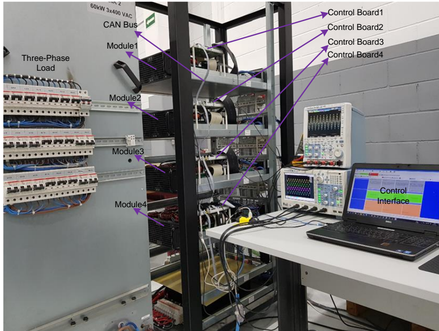
Figure 1- 6 Modular UPS platform in Salicru.
