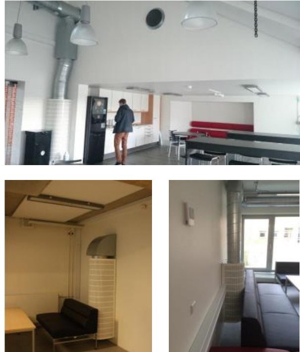
Figure 4 Misuse of displacement ventilation
