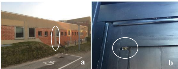
Figure 3 Uninsulated concrete beams (a) and cracks in window frame (b)
