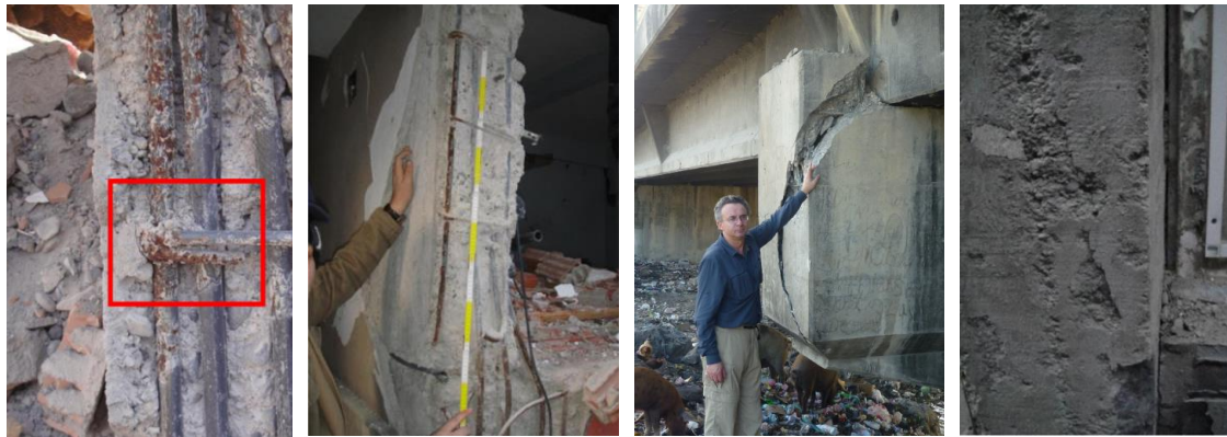
Figure 1. Common deficiencies of substandard RC buildings a) improper hooking and usage of plain bars, b) pull out failure and c) low concrete quality.
