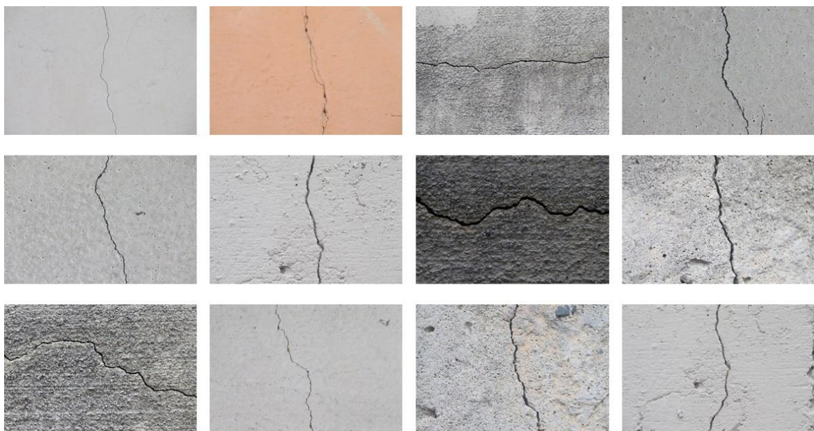
Fig. 4.3 Example crack images in different conditions.
