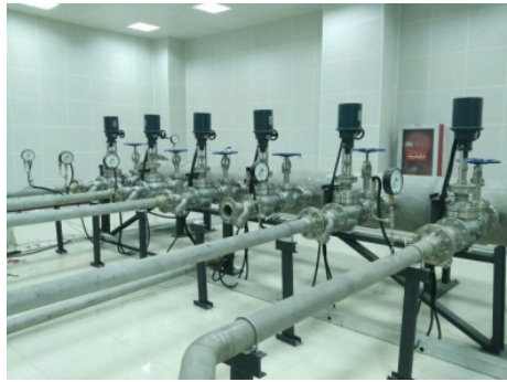
Fig. 9. Pipelines and valves
