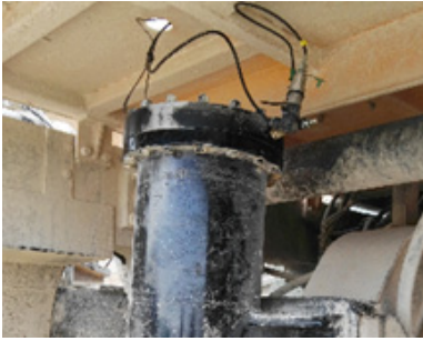
Fig. 5. Installation location of the acceleration sensor
