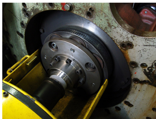
Fig. 1. Highly flexible coupling used for connection of ICE and electric generator
