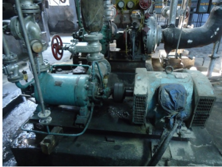
Fig. 15. Photograph of boiler feed pump
