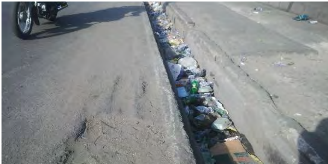
Plate 9.27: Drainage littered with refuse on Warehouse Road Source: Author, 2018
