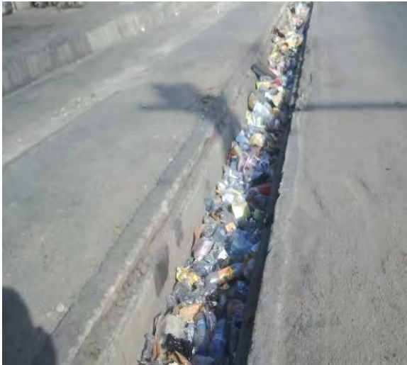
Plate 9.25: Blocked drainage on Creek Road Source: Author, 2018
