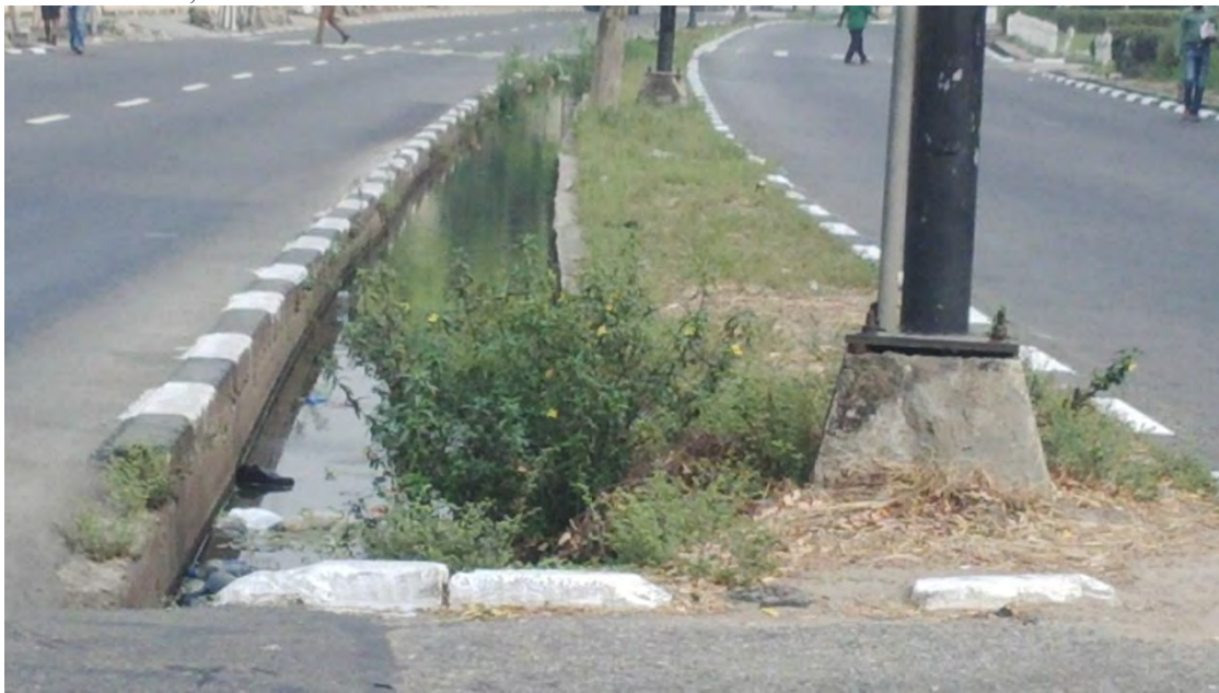
Plate 9.37: Poorly constructed and maintained drainage on Ahmadu Bello Way, Victoria Island
