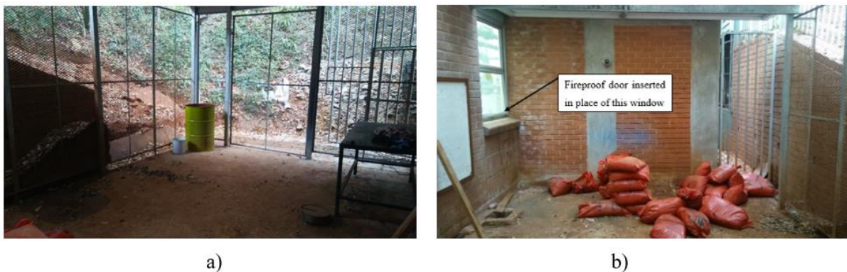
Figure 3.1: (a) Test facility prior to completion and (b) location of access to existing laboratories
