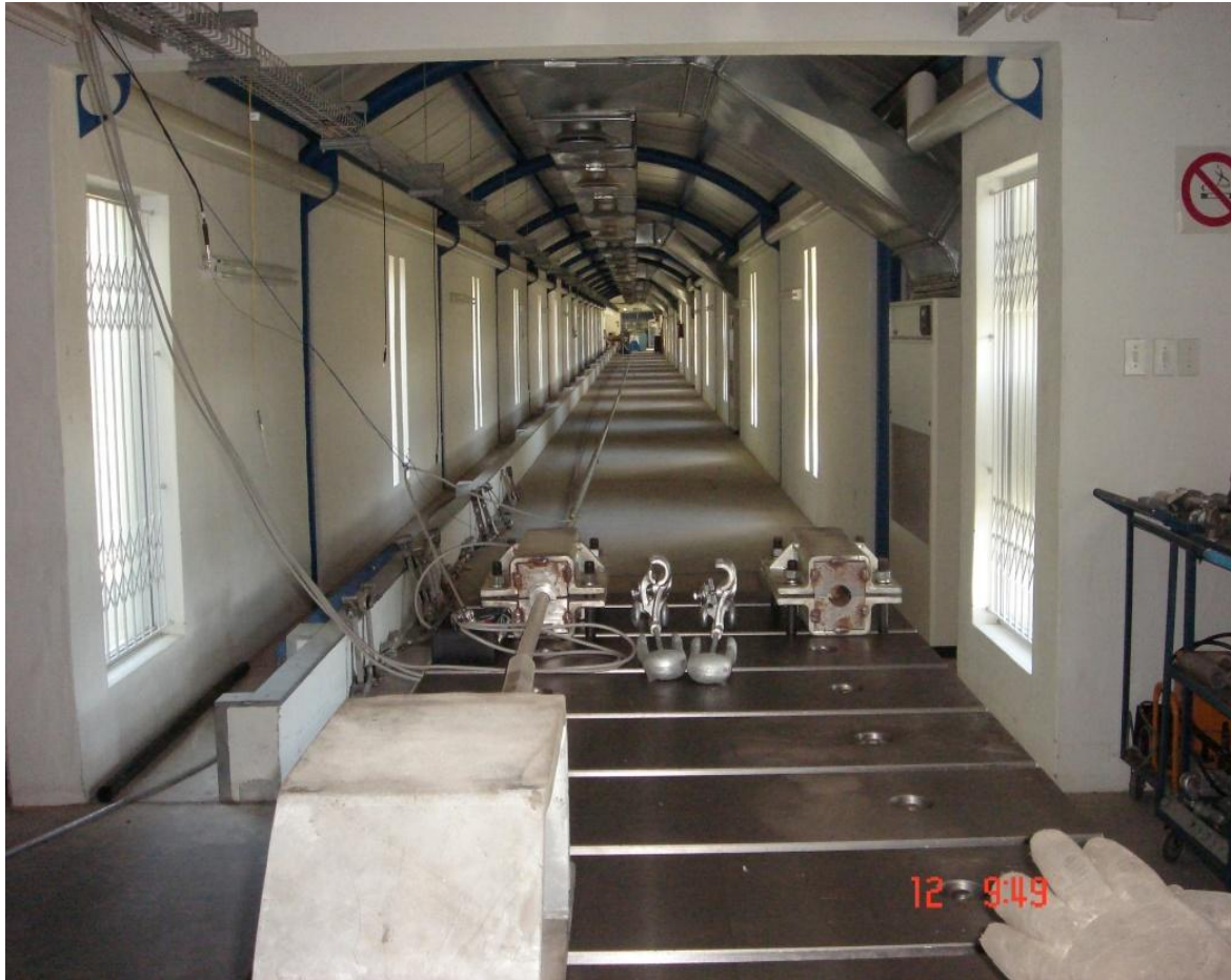
Figure 5.1 Facility tunnel and single span conductor at the VRTC
