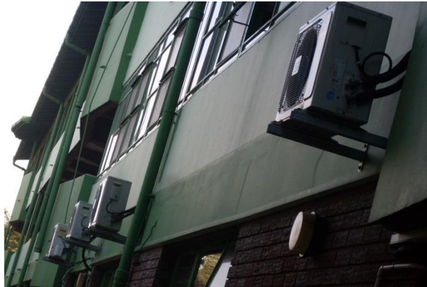
Figure 5.10: Air-conditioning units which serve only selected rooms
