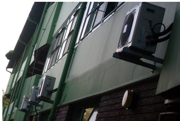
Figure 5.23: Air-conditioning units in spaces deemed important
