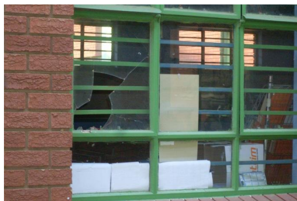
Figure 5.9: Broken windows on a classroom
