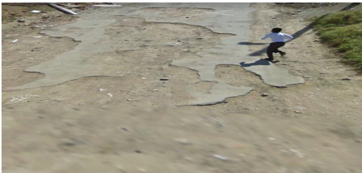
Plate 5.8: Damaged roads within Ikwezi Township
