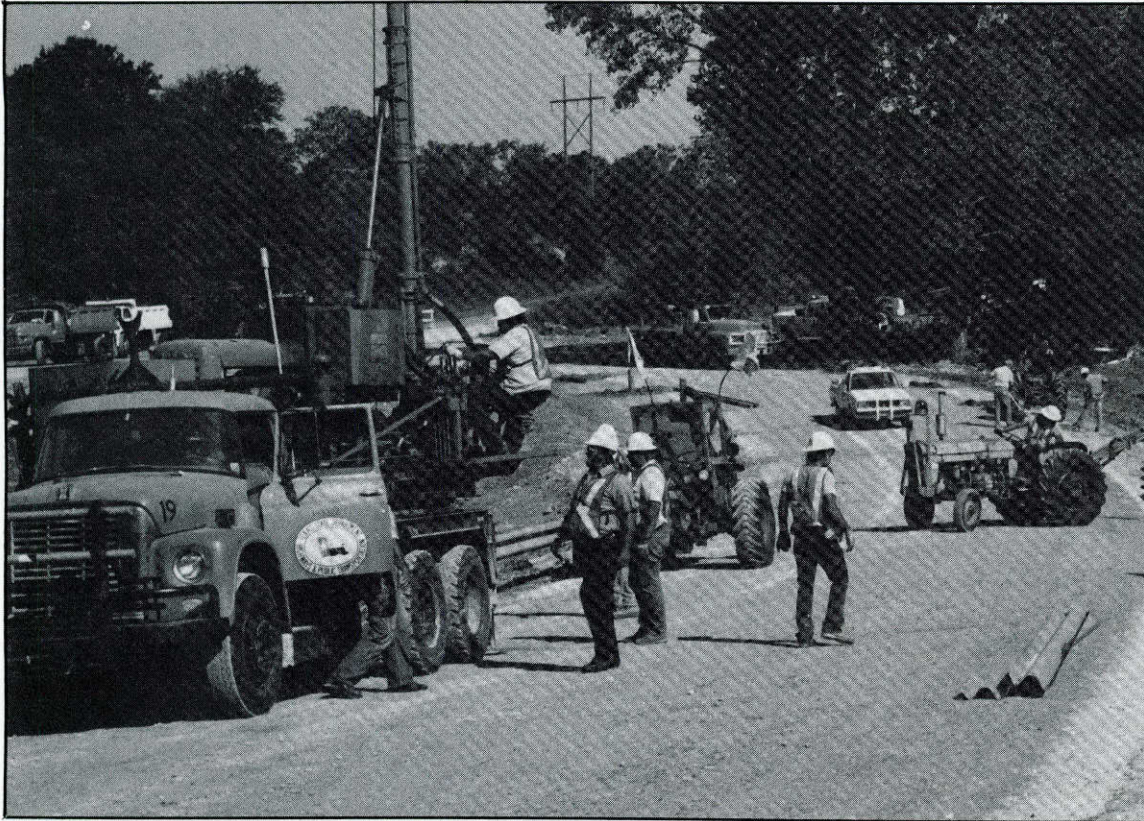
A Paris District crew installs guardrails along a US 75A detour. The project was paid for with private funds to hasten construction of the detour around the flood-devastated roadway.
