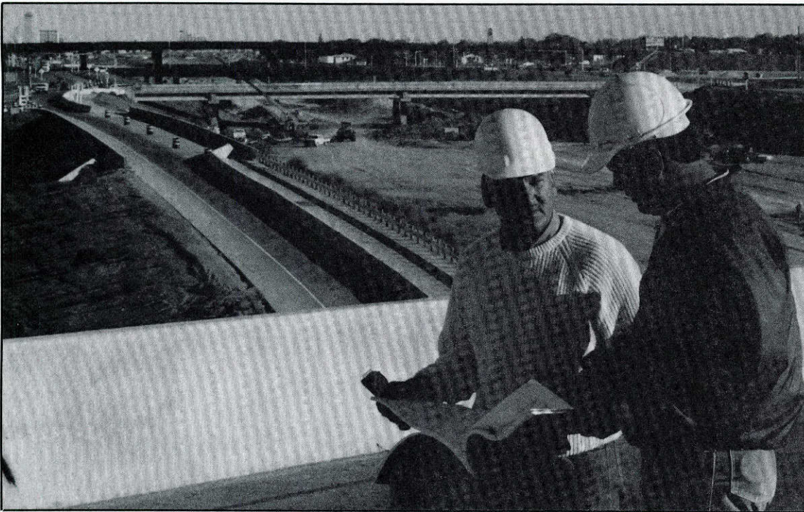
Reviewing Interstate 27 construction plans are Fred Long and Lewis Gamboa, inspectors for the project.
