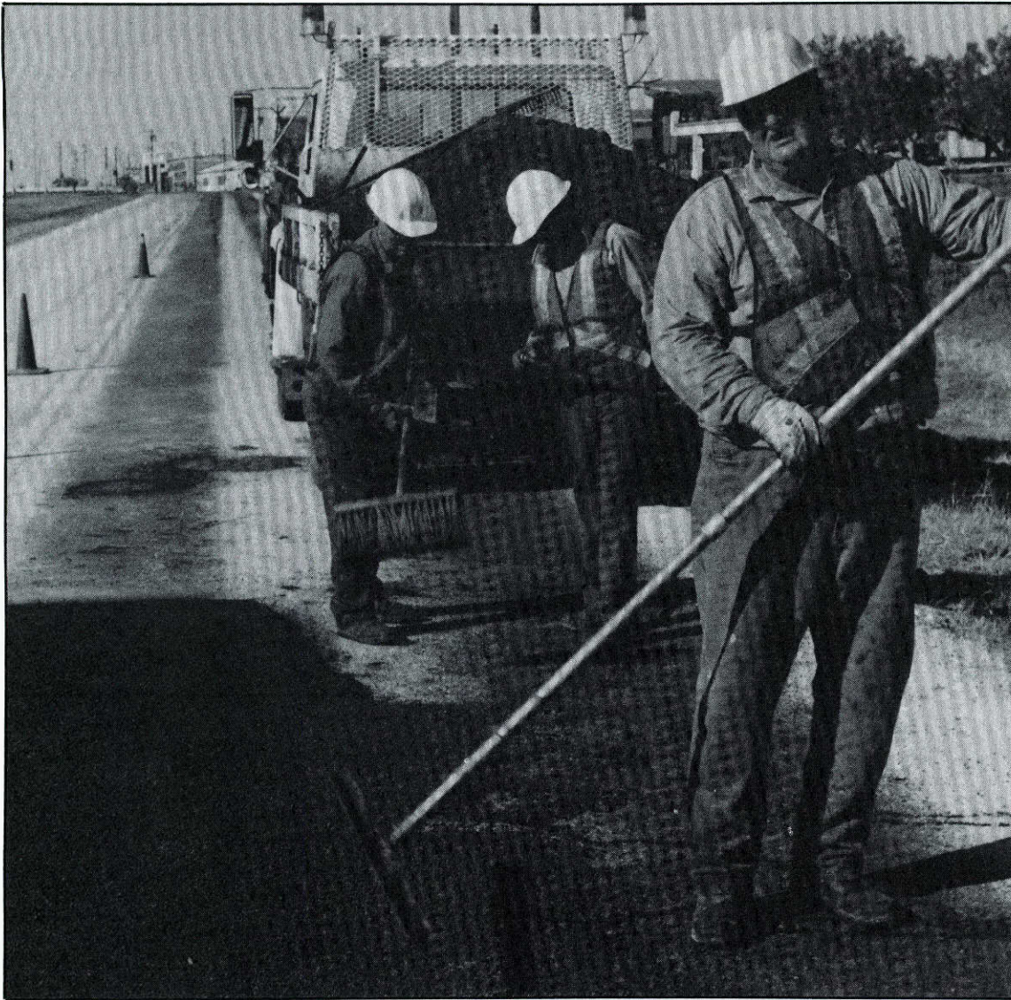
Taylor County maintenance employees patch a section of the Interstate 20 north frontage road at Tye.
