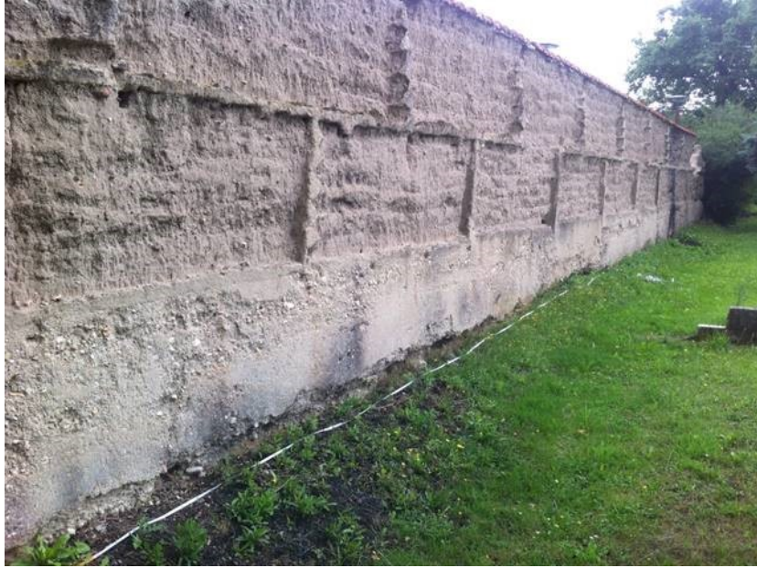
Figure 2: Damage (loss of surface material) to a pisé wall in Précieux in the Loire Department, France, due to exposure to direct rainfall. Photograph: Nicolas Meunier
