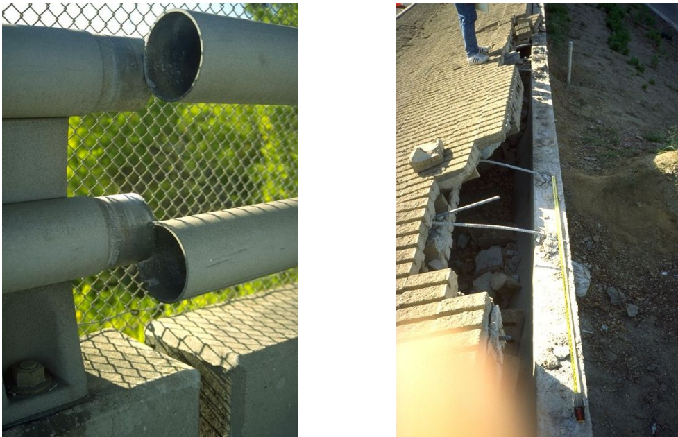
Fig. 2.26: Seismic damage to non-structural elements of bridges
