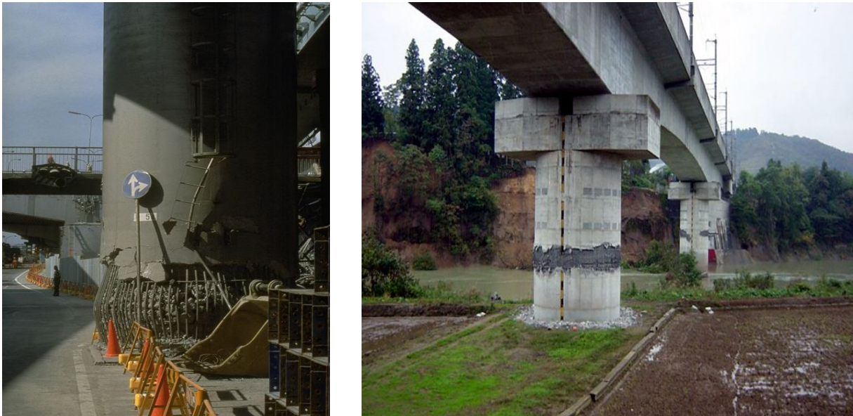
Fig. 2.9: Flexural damage to bridge piers
