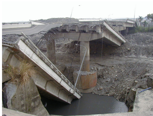
Fig. 2.5: Unseating of Ming-Chu bridge during Chi-Chi earthquake 1999 (Source: EERI)
