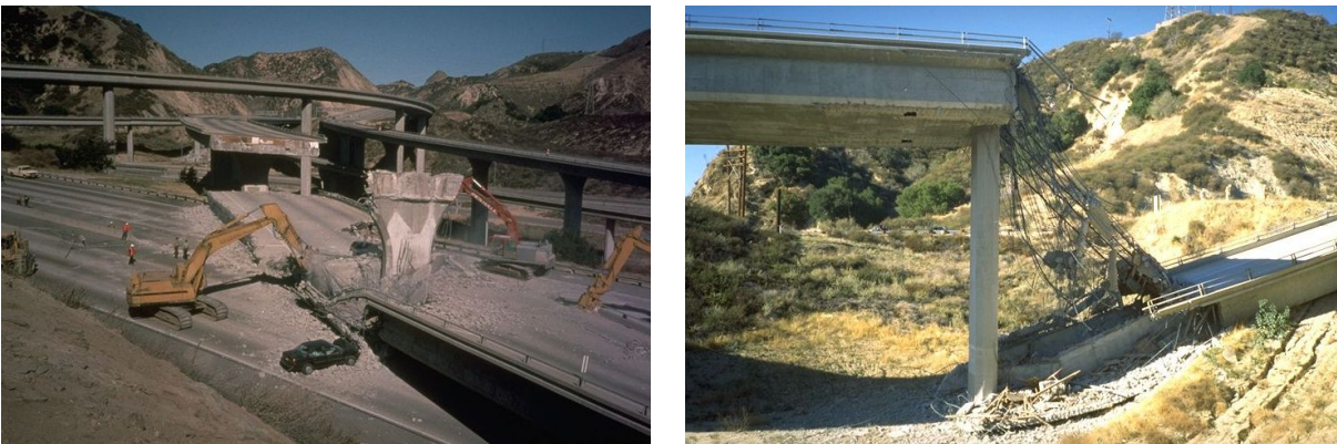
Fig. 2.4: Unseating of I-5 Highway 14 during Northridge earthquake 1994 (Source: Mark A. Aschheim, NISEE)
