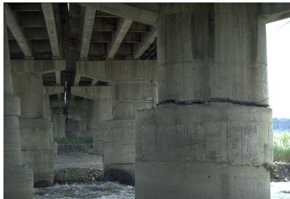
Fig. 2.12: Onset of sliding shear in pier of Wu-Hsi bridge during the Chi-Chi earthquake 1999 (Source: Jack P. Moehle, NISEE)
