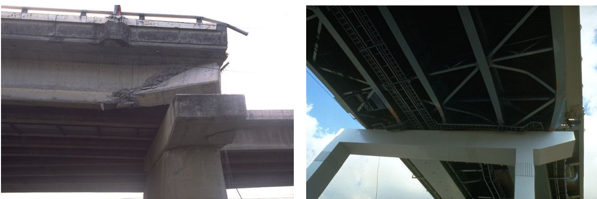
Fig. 2.23: Damage to the webs of superstructure girders
