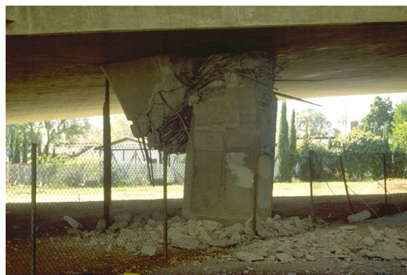
Fig. 2.11: Loss of shear capacity in heavily damaged plastic hinge region Mission Gothic bridge after Northridge earthquake 1994 (Source: Graham C. Archer, NISEE)
