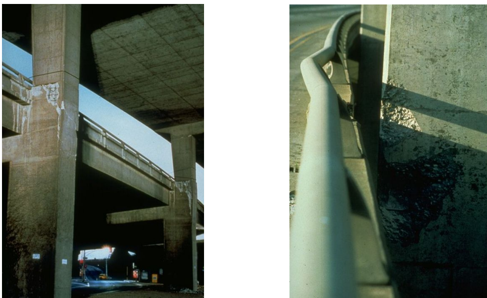
Fig. 2.25: Damage due to pounding in the transverse direction at Southern Freeway Viaduct after Loma Prieta earthquake 1989 (Source: NISEE)
