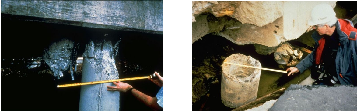
Fig. 2.19: Damage to piles left: Pile at Struve Slough Bridge after Loma Prieta earthquake 1989 (Source: NISEE), right: Sheared off piles after Kobe earthquake 1995 (Source: NISEE)
