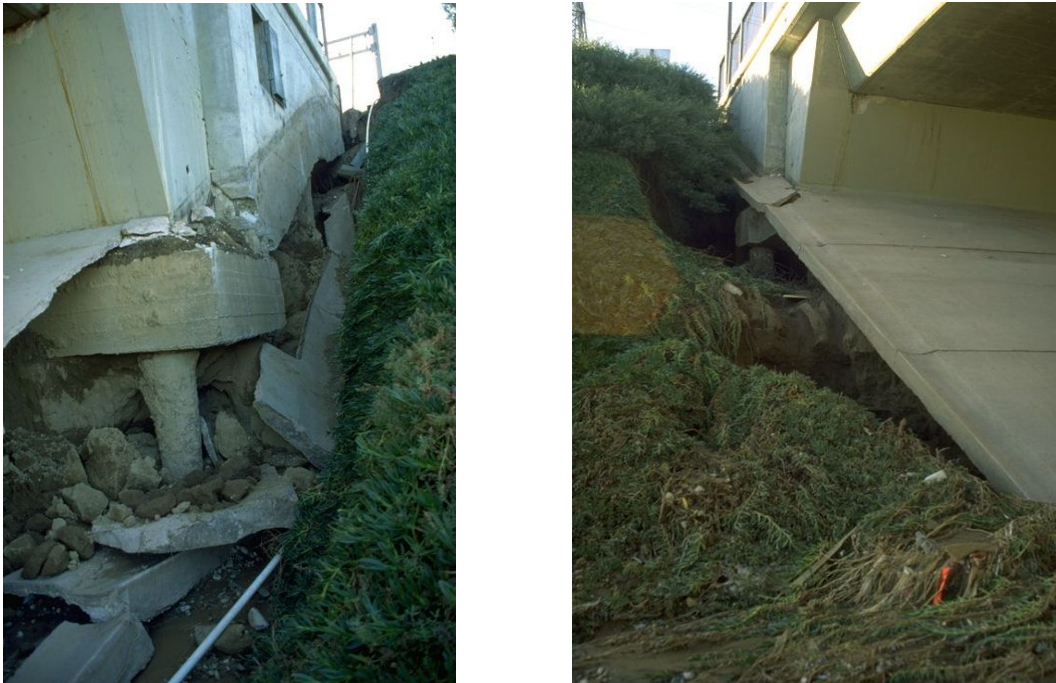
Fig. 2.14: Abutment movement at Highway 118 during Northridge earthquake 1994 (Source: Graham C. Archer, NISEE)
