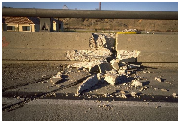
Fig. 2.24: Local damage due to pounding at an expansion joint of I-5/Santa Clara River after Northridge earthquake 1994 (Source: Mark A. Aschheim, NISEE)
