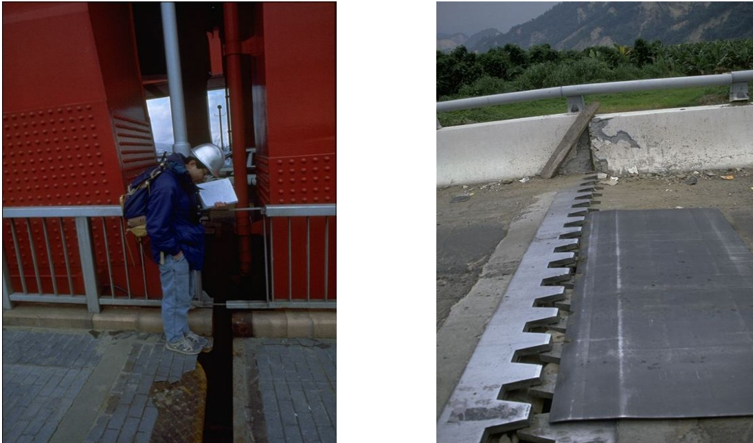
Fig. 2.18: Damage to expansion joints left: after Kobe earthquake 1995 (Source: Christopher R. Thewalt, NISEE), right: after Chi-Chi earthquake 1999 (Source: unknown)
