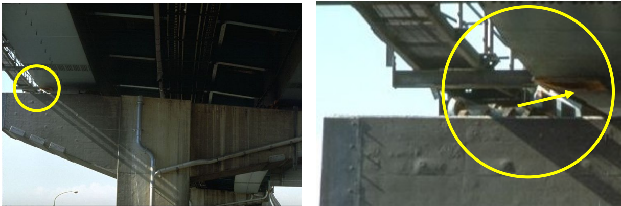
Fig. 2.7: Bearing failure and subsequent transverse shift at pier of Hanshin Expressway during Kobe earthquake 1995 (Source: Christopher R. Thewalt, NISEE)
