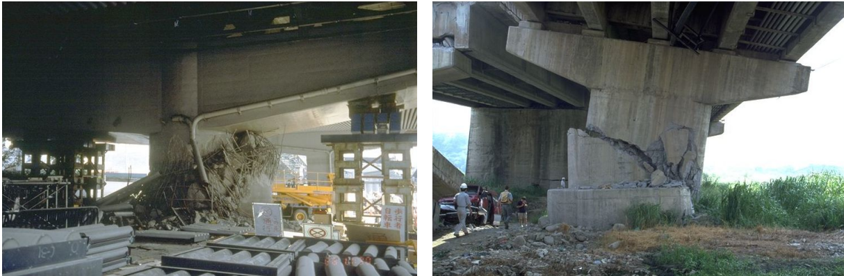
Fig. 2.10: Shear failure of squat bridge piers left: Hanshin Expressway Pier 57 after Kobe earthquake 1995 (Source: Christopher R. Thewalt, NISEE), right: Wu-Hsi bridge after Chi-Chi earthquake 1999 (Source: Jack P. Moehle, NISEE)
