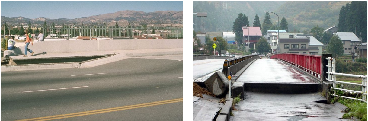
Fig. 2.21: Settlements of the embankments left: Abutment backfill after Northridge earthquake 1994 (Source: NISEE), right: Embankment after Niigata-Ken earthquake 2004 (Source: Mitsutoshi Yoshimine, NISEE)
