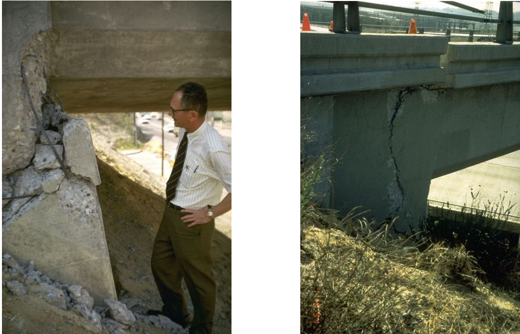
Fig. 2.16: Structural damage to abutments left: I-5/I-210 Interchange after San Fernando earthquake 1971 (Source: Karl V. Steinbrugge, NISEE), right: I-5/I-210 Interchange after Northridge earthquake 1994 (Source: NISEE)
