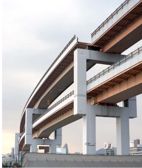
Fig. 2.6: Large transverse shift of superstructure after Kobe earthquake 1995 (Source: NISEE)
