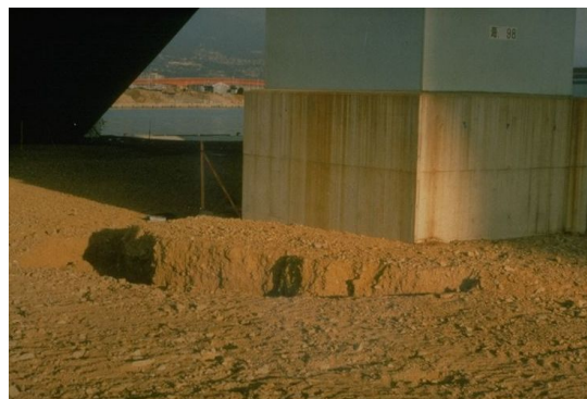
Fig. 2.20: Soil liquefaction around pier foundation at Nishinomiya bridge after Kobe earthquake 1995 (Source: Christopher R. Thewalt, NISEE)
