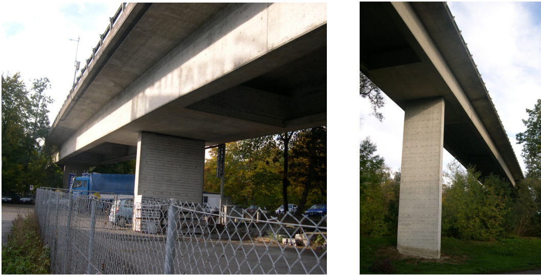
Fig. 2.42: View of Viadukt Mühle Rickenbach in SG left: Short pier P1 close to the north end of the bridge, right: Long pier P3 in the center of the bridge
