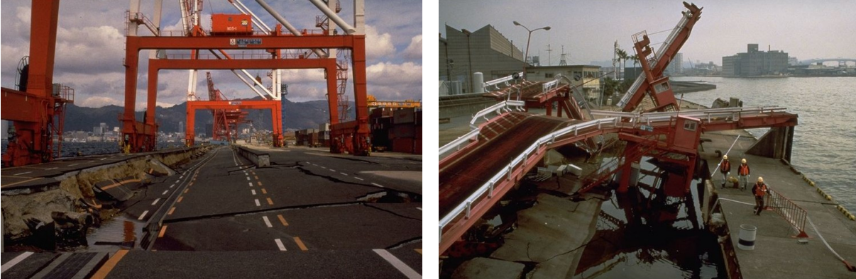
Fig. 2.54: Damaged port of Kobe after the earthquake in 1995
