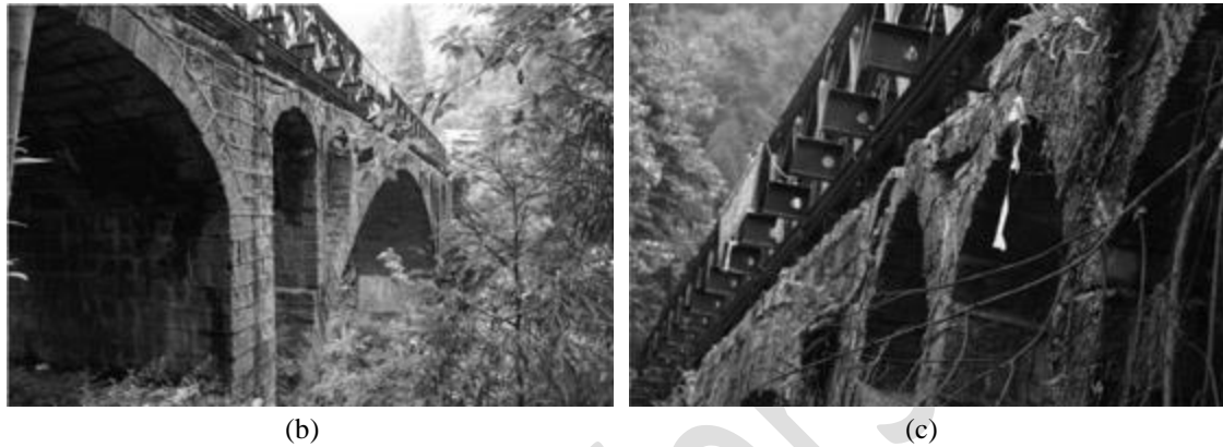
99 Figure 2 - Multi-span bridges: (a) overall longitudinal arch-pier mechanism (AP-L); (b, c) damage to the 100 Guantong Bridge, China, due to large displacements in the longitudinal direction in the 2008 Wenchuan 101 earthquake (after [13]). 102 103 104
