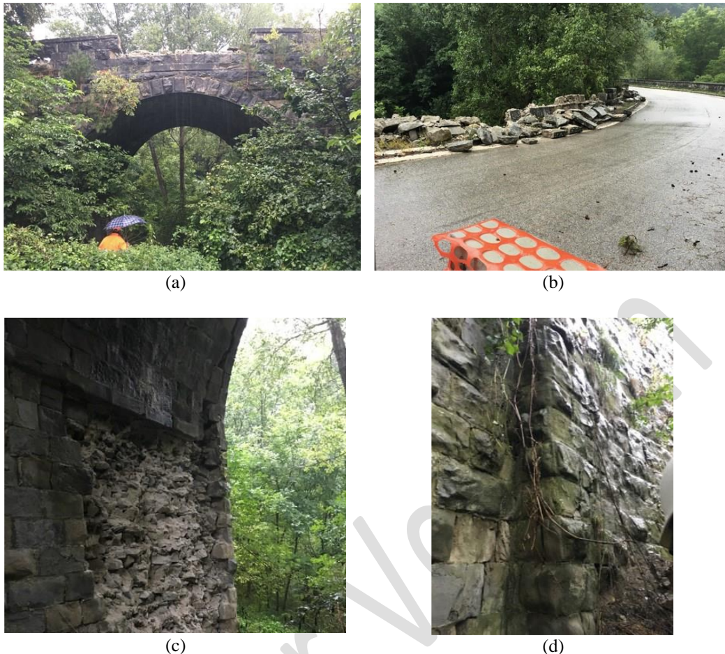
414 Figure 13 - Three-span masonry bridge along the “Trisungo-Tufo” route (42.73538 N, 13.253655 E): (a, b) 415 out-of-plane collapse of the parapet over the central arch; (c) spalling and (d) cracking of some masonry 416 elements.
