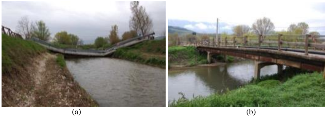
250 251 252 Figure 8 - Bridge damage in the 209 L'Aquila earthquake, Italy: (a) bridge collapse near Fossa; (b) deck 253 failure near Onna (after [26]). 254
