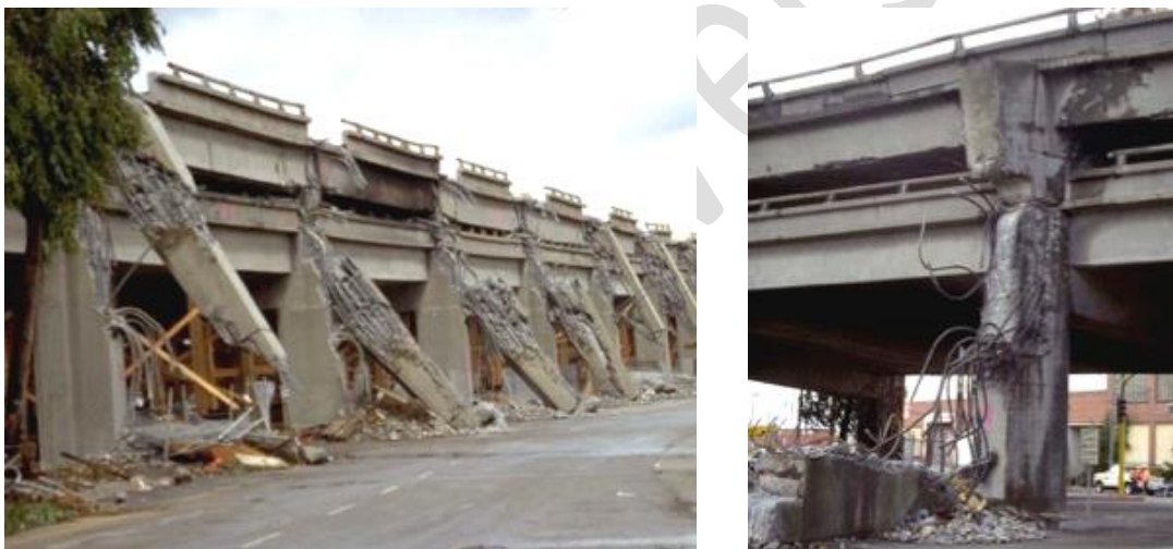
190 Figure 6 - Shear failure of pier-bent cap joints, and anchorage failure of beam longitudinal bars of the 191 Cypress viaduct in Oakland, California, during the 1989 Loma Prieta earthquake (courtesy of NISEE). 192 193
