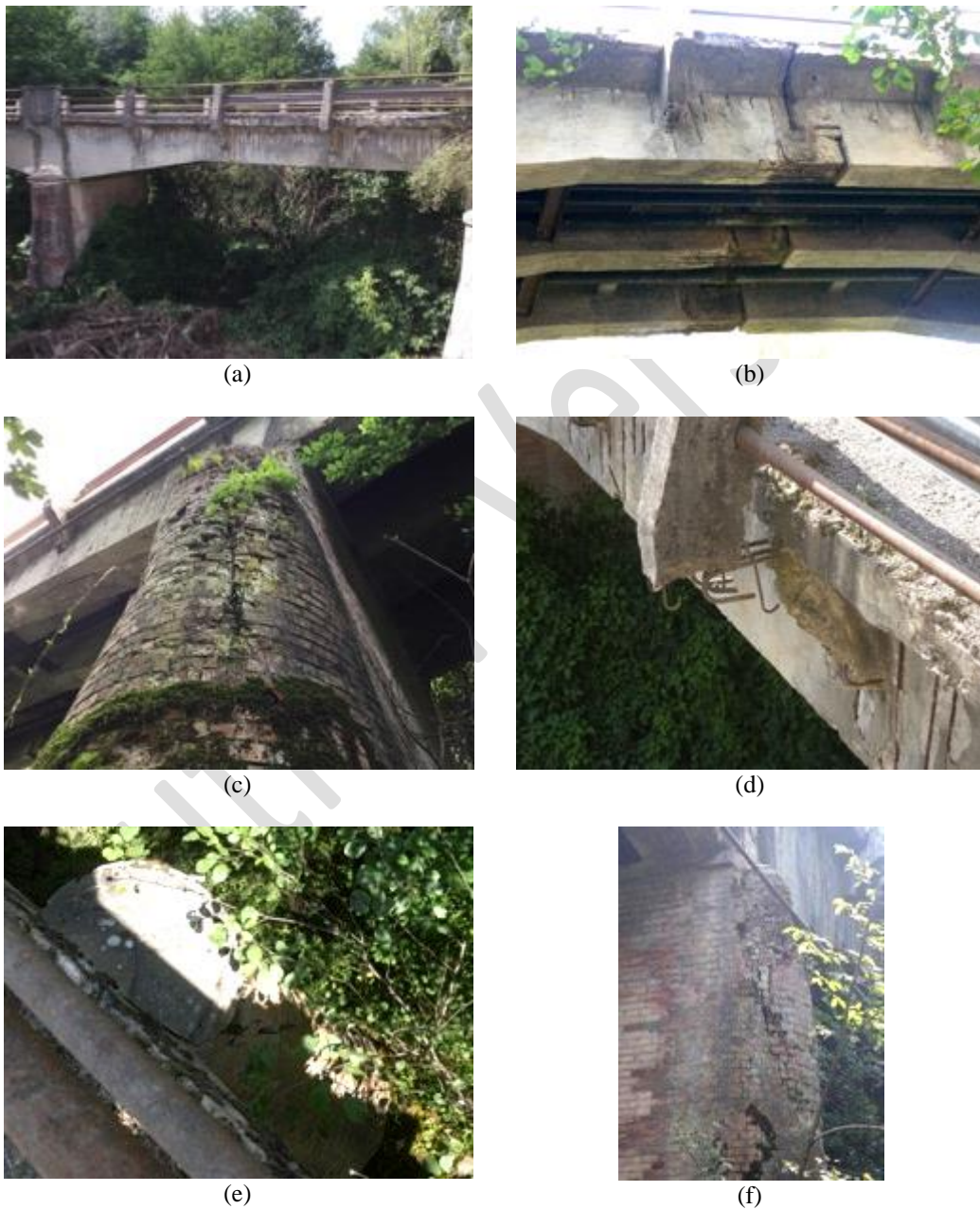
450 Figure 14 - “Rosa” reinforced concrete and masonry bridge (42.623178 N, 13.250428 E): (a) elevation view 451 of the North-East bay; (b) degradation of the reinforced concrete Gerber girders; (c) degradation of the 452 masonry piers; (d) pre-existing damage of a parapet connection to the deck; (e, f) cracking and partial 453 collapse of the exterior brick leaf of the piers. 454 455
