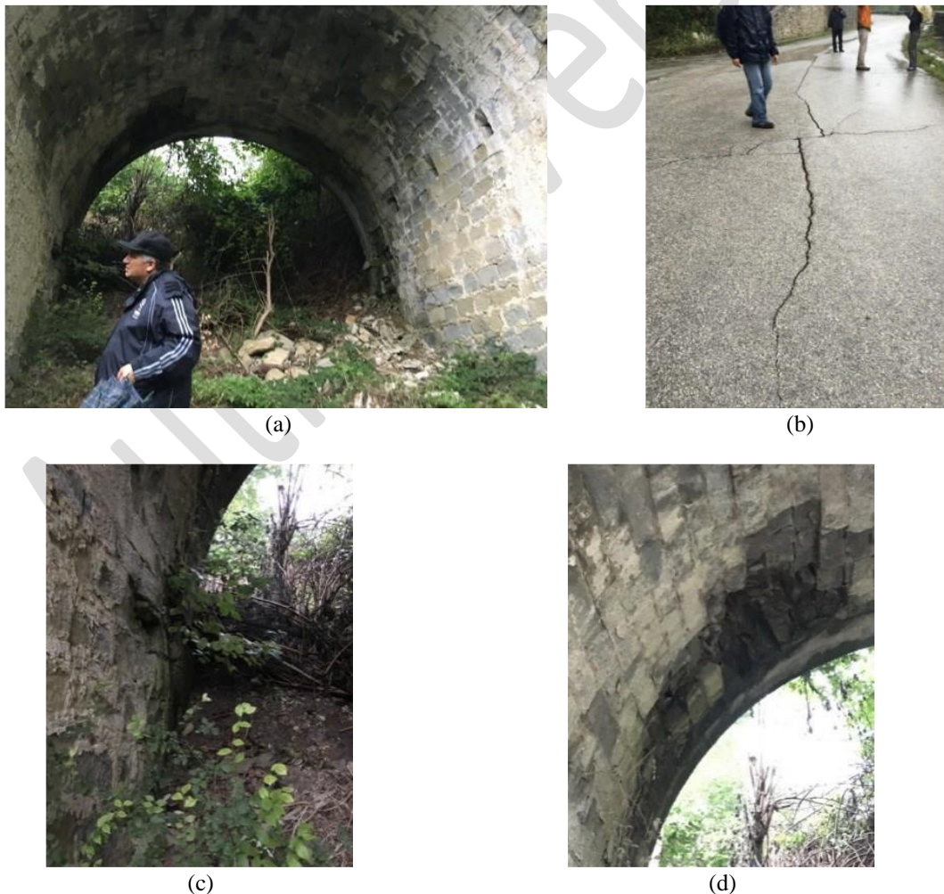
411 Figure 12 - Single-span masonry bridge along the “Trisungo-Tufo” route (42.735981 N, 13.254862 E): (a) 412 view of the bridge; (b) damage on the road pavement; (c) spalling of the outer leaf of the abutment; (d) 413 spalling of the intrados of the vault.
