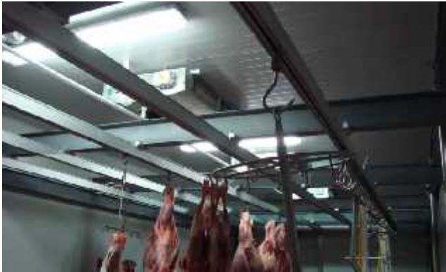
Figure 2 Evaporators location inside cold room n. ° 1.
