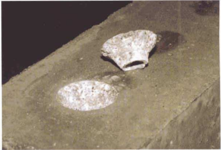
Figure 11 - Failure type is observed for validation of result.
