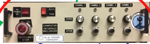
Computer Interface Enclosure
