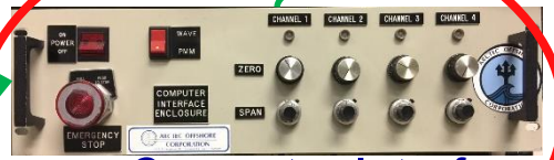
Computer Interface Enclosure
