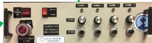
Computer Interface Enclosure
