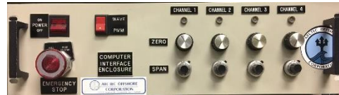
Computer Interface Enclosure
