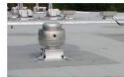
Securing Small Rooftop Equipment to Curbs: Attach stacks, exhaust fans and air intakes to the curb with corrosion resistant fasteners not exceeding 6in. on centers between the equipment, transition pieces, and the roof curb. (Ref. 1)
