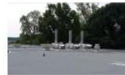
Overhanging Trees: Tree located near or above structures should be trimmed periodically to prevent damage to the structure and reduce the amount of organic debris on rooftops which pose drainage issues and potential fire hazards.
