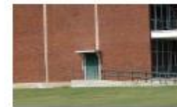
Attached Structures: Periodically check connections of carports, canopies and porches to prevent wind related damages: 1) Connections between tops of columns and roof. 2) Connections between bottom of columns and foundation. (Ref. 6)
