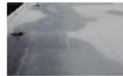
Drainage Issue: Evidence of water ponding on rooftop
