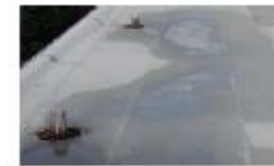
Drainage Issue: Roof drain is clogged, preventing adequate drainage.
